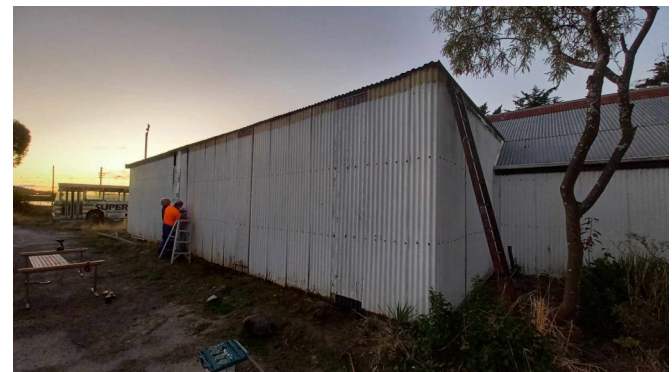
Top 3 photos: Showing the progress of the exterior cladding with the building wrap being installed and then the iron going back on finally as the sun sets. Photos by Alan Hinman.
