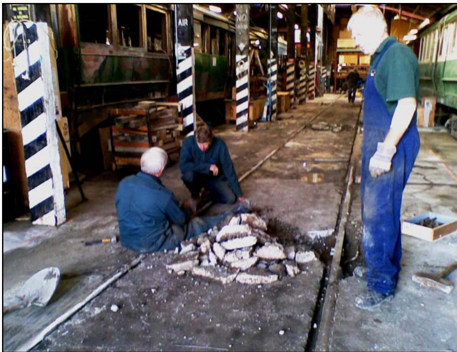
Society President Graeme Belworthy and Bruce Maffei replace rusted tracks bolts on the fishplates of the rail joints on main running road in Tram Barn 1 while Track Office Ken Henderson looks at the mess they are making.
