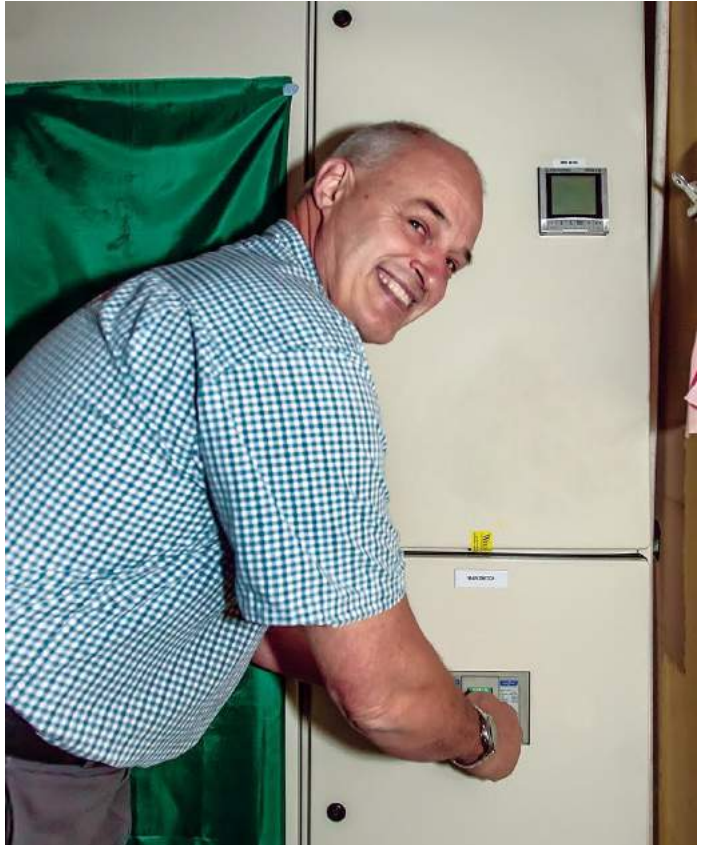
ABOVE: It's On! Andrew McLean (Bremca) officially turns on the new THS Switchboard, 16/03/2017/.
